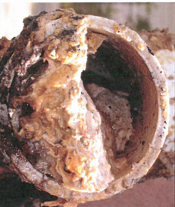
A sewer pipe clogged with FOG (Fats, Oils & Grease)
