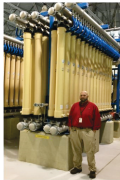
Grade IV operator Keith Kelly stands next to filter rack #5 at the Jerry Plott Plant
