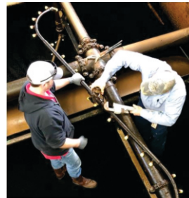
Maintenance workers at the Ed Love Plant repair a surface wash agitator
