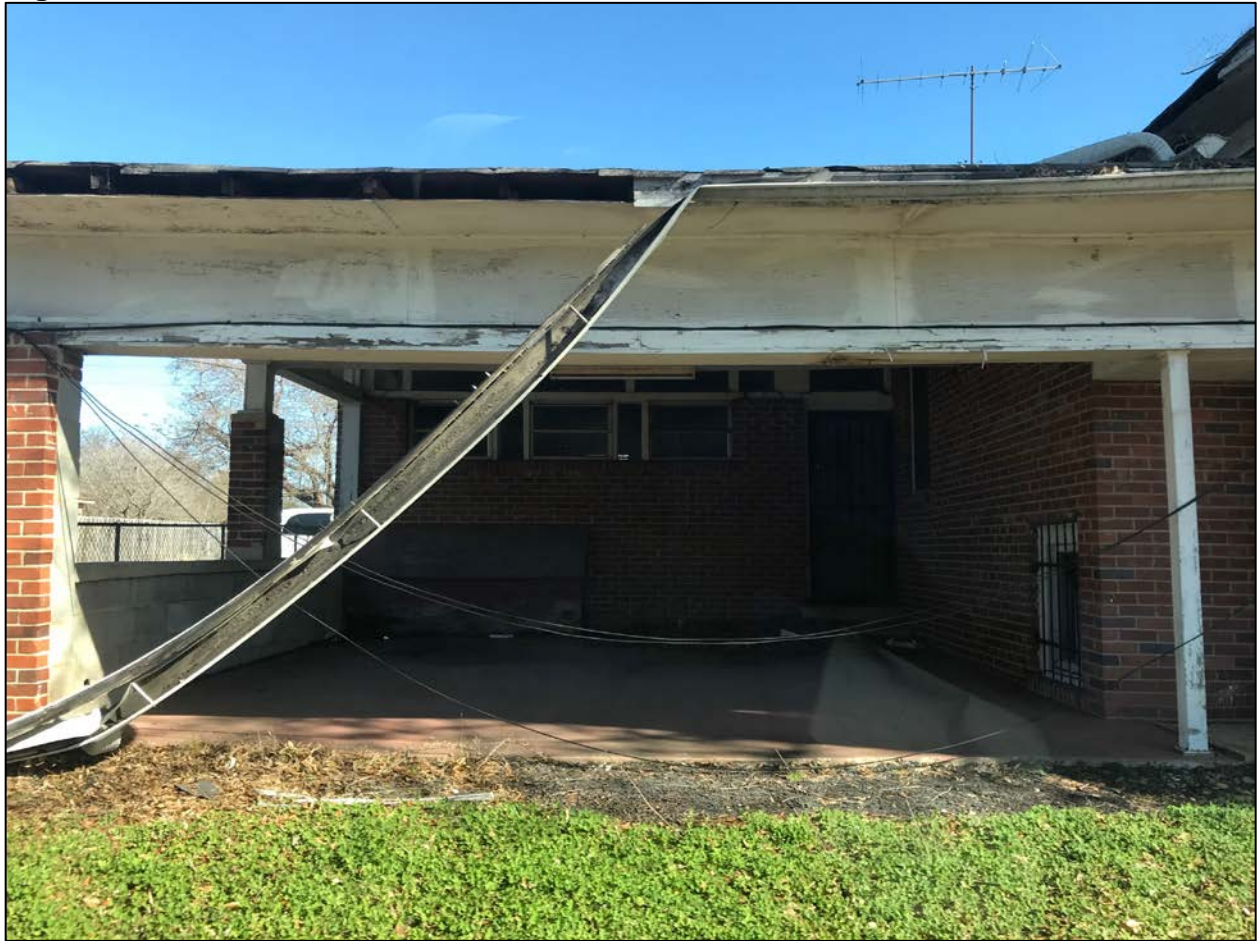
Figure 7. Abandoned Home with Fallen Gutter and Power Lines
